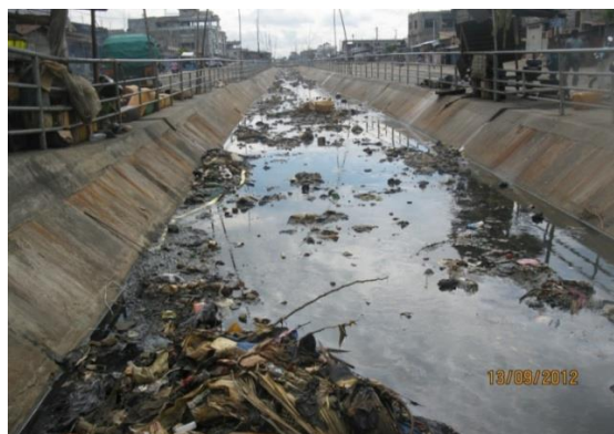
Photo 1 : Open gutter obstructed by DSM at Agbato
