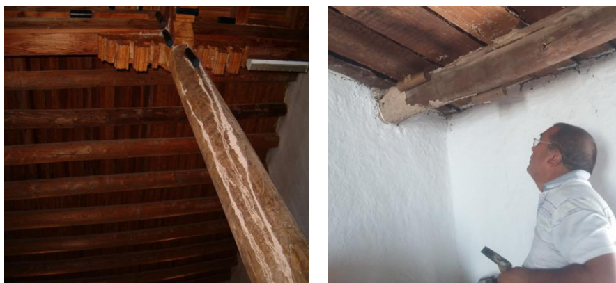
Figure 3. Installation of food-bait containers on A- the columns that termites damaged in Juma mosque and B- beams that termites damaged on residential buildings of the Ichon-Kala Nature Museum in Khiva, Khorezm region.
